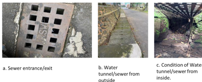
Figure 4. The conditions of the SWCU sewer before testing since the robot was not covered with waterproof
