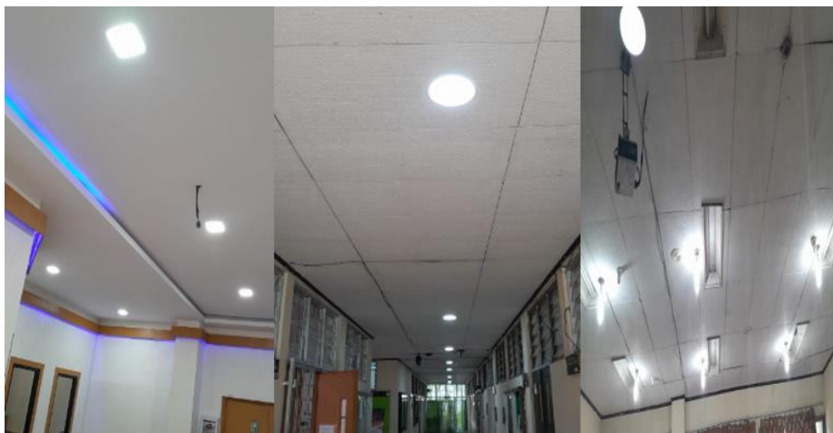
Figure 2. lighting served by solar panels
