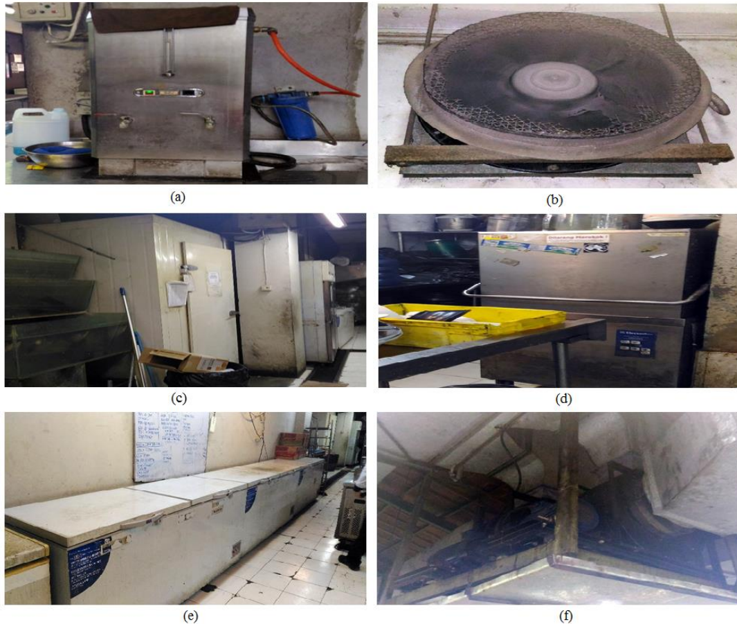
Fig. 1. Electrical Appliances at F&B Department: (a) Water heater, (b) Exhaust Fan, (c) Walk in chiller, (d) Dishwasher, (e) Under chiller, (f) Blower Wheel
