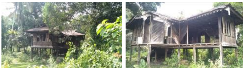
Figure. 3. (Left) View from the South. Figure. 4. (Right) Damage to Building Components
