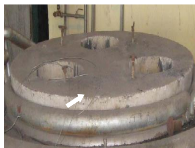
Figure 6. Castable refractory (refractory cast cement) electric arc furnace
