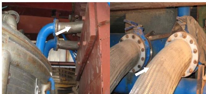
Figure 7. Electric arc furnace roof cooling hose
