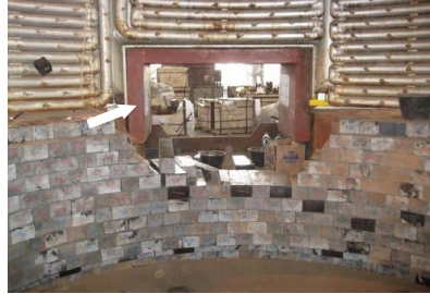
Figure 4. Slag electric arc furnace door
